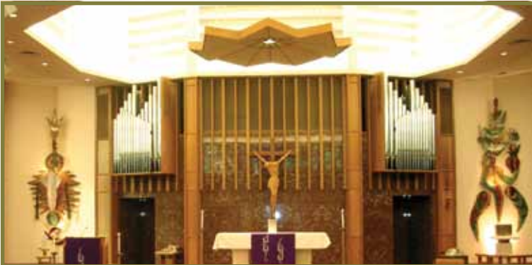
New, energy-efficient lighting has been installed in Our Lady of Grace church in Scott Township.
